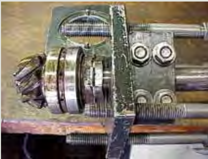
#11. Close up view before puller tool is removed. The four nuts and bolts holding the clamping device to the drive shaft are to be loosened and the device slid off the drive shaft.
